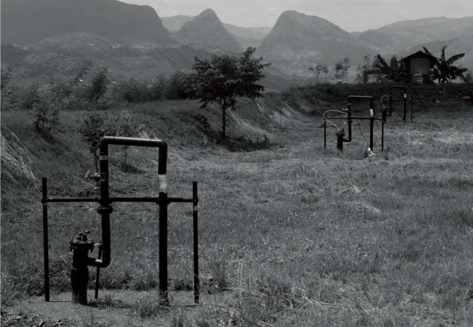
A network of pipes collects methane gas from the decomposing garbage buried in the landfill. The collected gas is then converted by the Montalban power plant into electricity. But there would be negligible gas if garbage were segregated, as required under an existing law. (By SONNY YABAO)
