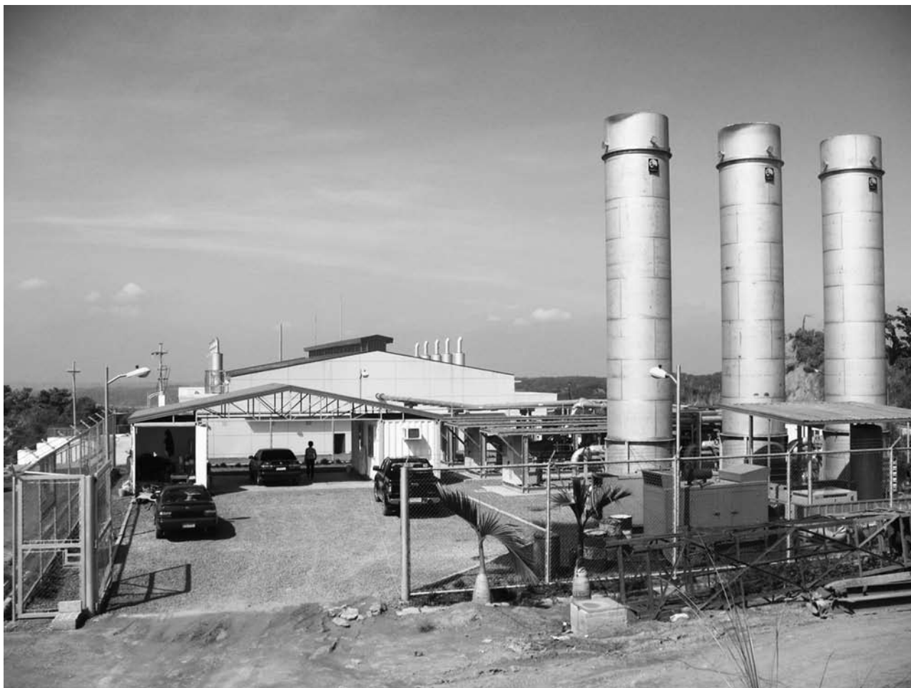
The Montalban methane power plant sits atop one of the foothills of the Sierra Madre range, in Rodriguez (formerly called Montalban) town in Rizal province. (By ECOWASTE COALITION)
